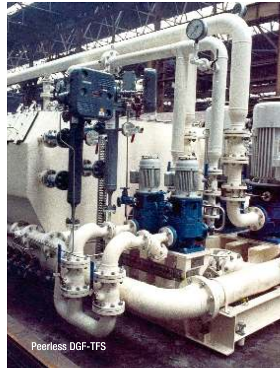
Skid assembly for DGF pumps with free-gas vent vessel for large DGF units
