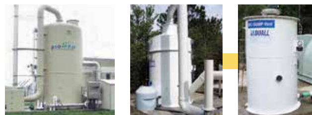
Biotrickling Filter Removing Odors
