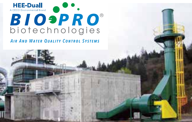
Biofilter Removing Hazardous Air Pollutants (HAPs)
