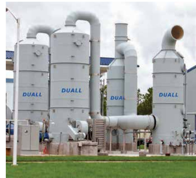
DUALLast® Degasifiers, Scrubbers, Fans, and Stacks
