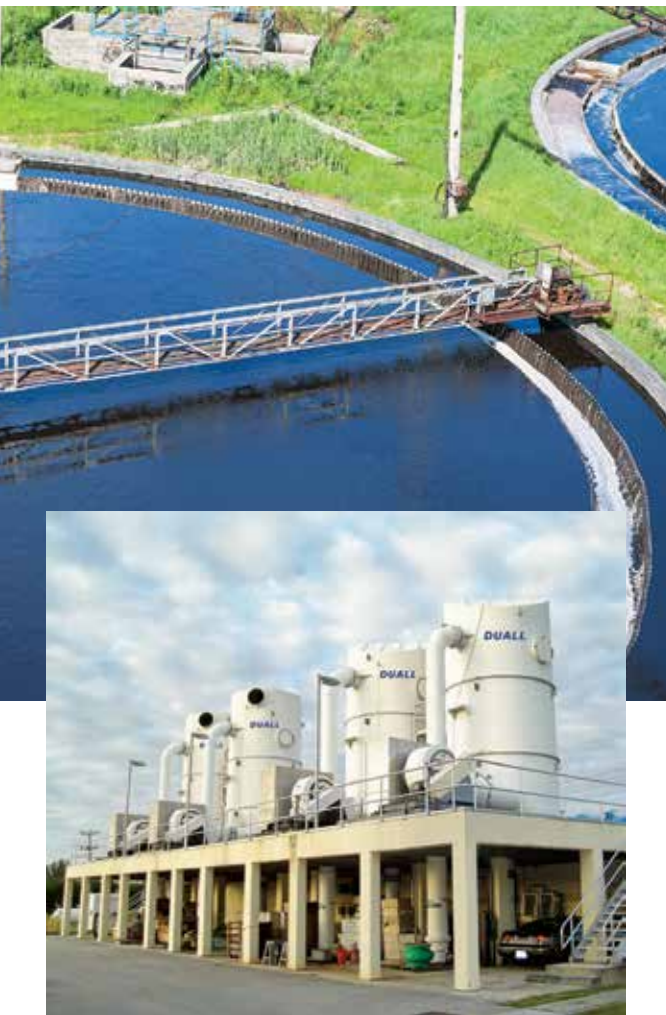
Water Production Plant with Degasifiers
