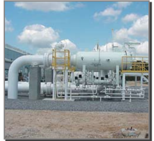
THIS PEERLESS FILTER-SEPARATOR IS INSTALLED AT A COMPRESSOR STATION IN NATURAL GAS TRANSMISSION SERVICE. THIS PEERLESS UNIT IS DESIGNED WITH A COST-EFFECTIVE FULL-DIAMETER CLOSURE.
