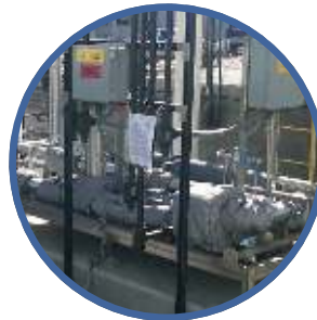
Urea or Ammonia Pump Skid
