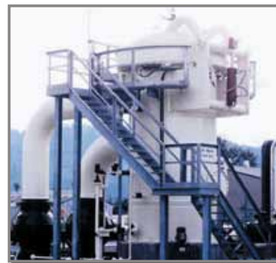
THIS ABSOLUTE SEPARATOR IS INSTALLED IN A METERING STATION IN CANADA. ITS 99" ID HOUSING UTILIZES A FULL DIAMETER, QUICK-OPENING CLOSURE.
