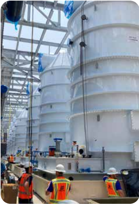
Vertical PP Scrubber
