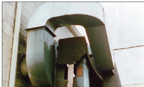
Figure 1. Example, ducts, short-radius elbows, and fan system effects that add to energy costs.
